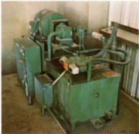
Remotely located, self-contained Power Unit.
