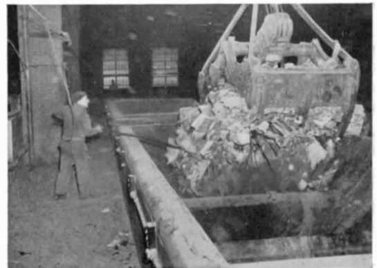
Crane feeding refuse into hopper of furnace. Note stoker chained to wall.
