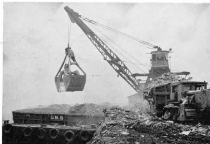
Unloading operations. Crane deposits refuse into conveyor wagons which transport refuse to bank of nearby landfill.
