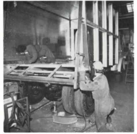
Craftsmen working on the horizontal discharge body of a 'Grenadier'. The body structure is mounted onto the chassis, the canopy and pressure plate mechanism being added later.
