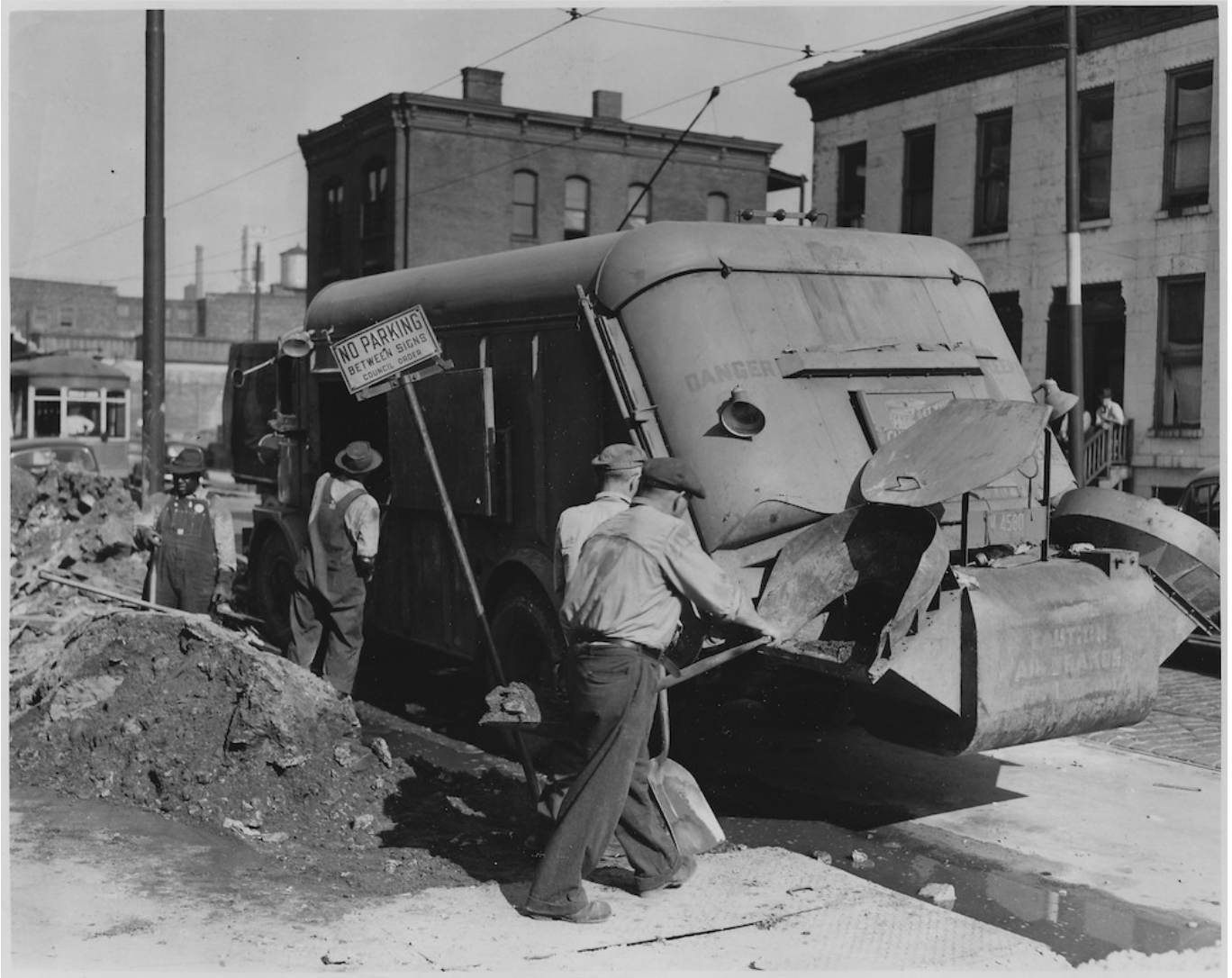
Crewmen loading demolition debris into a Heil Conveyor, which was capable of handling granular material as well as refuse
