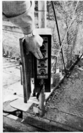
Remote controls are in box at discharge level.
