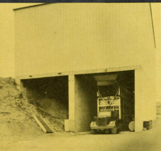
Compaction Trailer in position to receive refuse from above level. Note: In this particular installation, low cost, bi-level steel-and-concrete block structure, approximately 40' x 60', has been installed for all-weather use of system.
